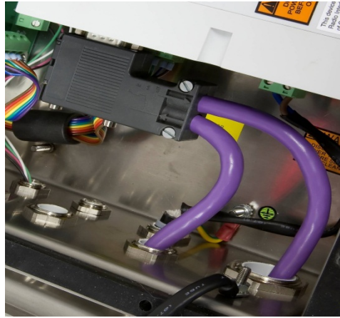
Figure 2-70: Original J-Box Enclosure PROFIBUS Cable Routing
