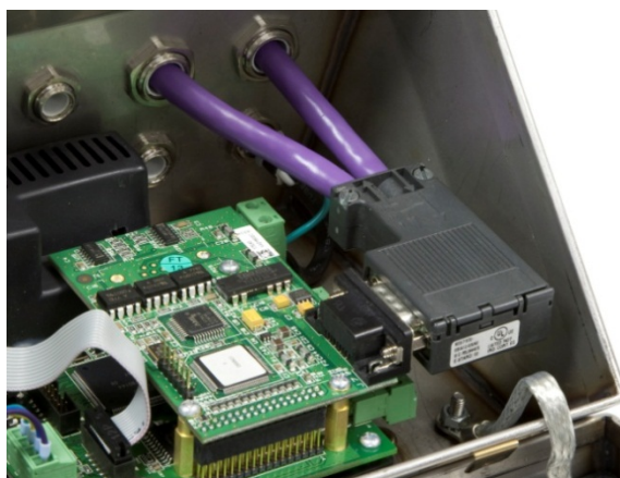
Figure 2-69: Harsh Enclosure PROFIBUS Cable Routing
