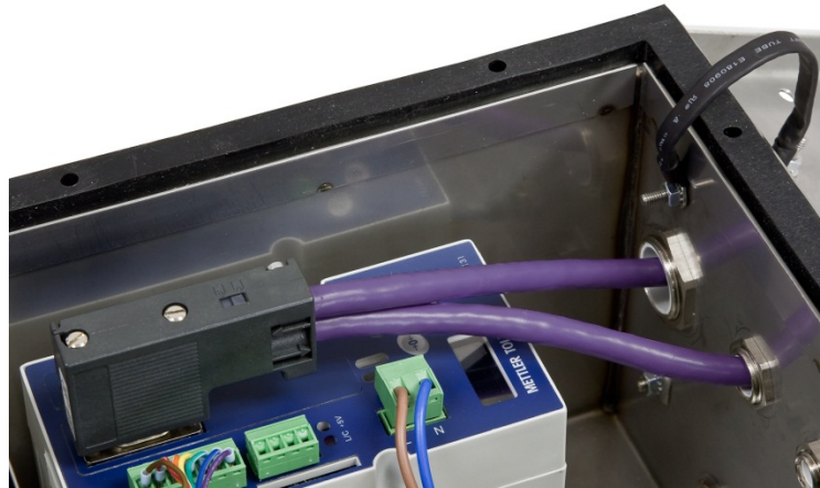
Figure 2-71: Updated J-Box Enclosure PROFIBUS Cable Routing
