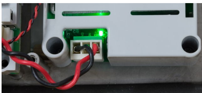
Figure 5-7: 12-VDC LED on Power Supply
