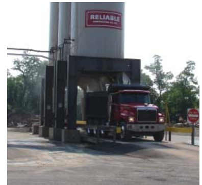
The truck scale and automatic filling system have helped increase plant throughput.
