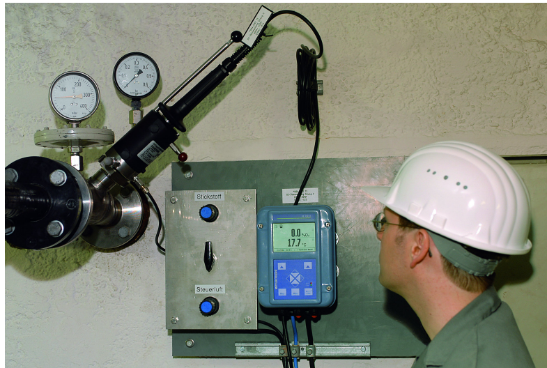
Direct oxygen measurement in the waste-gas manifold.
