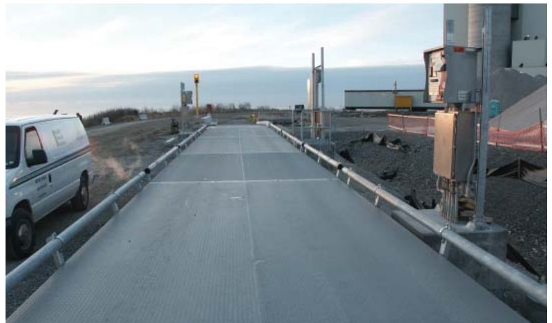
Unattended terminals allow drivers to weigh materials 24 hours per day, 7 days per week.
